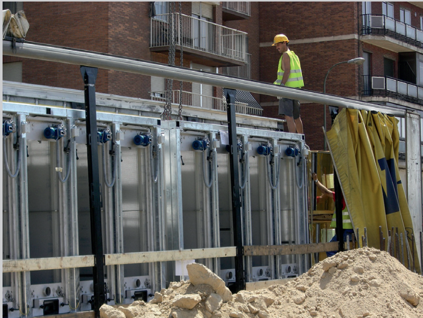
ECCO installation - Avenida Portugal
