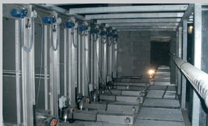
Automatic dampers for sectional cleaning
